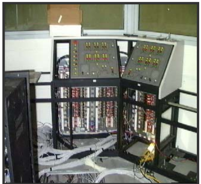
New Control Panel
