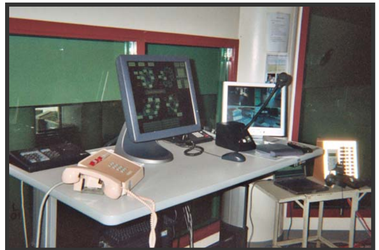
NEW CENTRAL CONTROL ROOM DISPATCH TYPE CONSOLE
