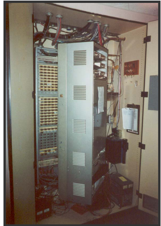
ORIGINAL EQUIPMENT CABINET
