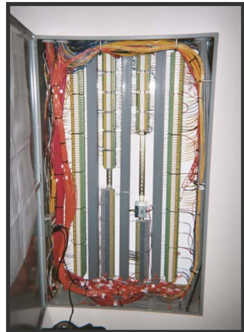
FINAL EQUIPMENT CABINET
